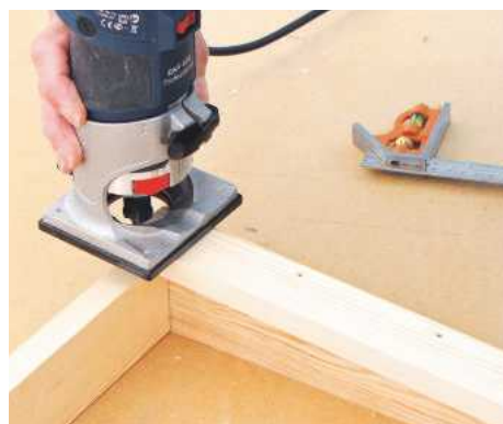
15 Sand arrises on shelves, then shape the ends of the support battens with a bearing-guided roundover router bit
