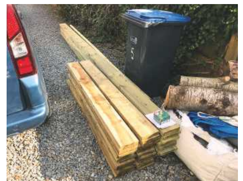
All building materials required were delivered just in the nick of time
