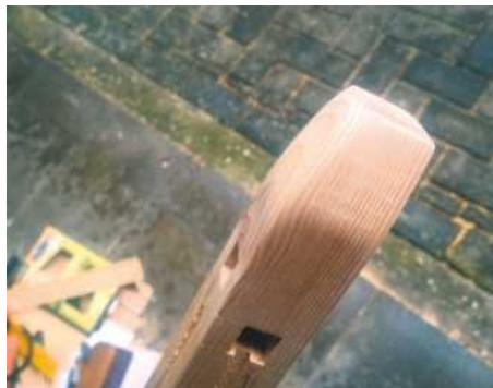
41 Use abrasives to reach the curve drawn on the bottom of each leg
