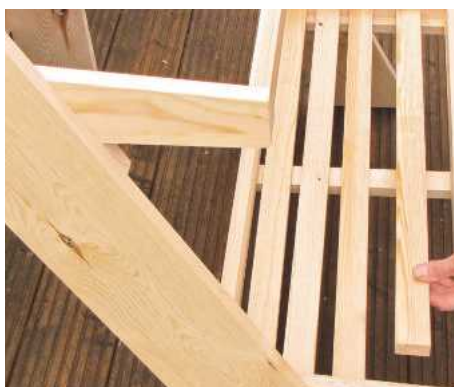
26 Saw remaining slats to length so they're a loose fit in shelf trays; sand and remove the arrises
