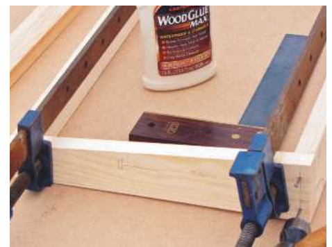
6 Spread glue and cramp shelf components together, leaving the ends slightly proud; punch heads below the surface
