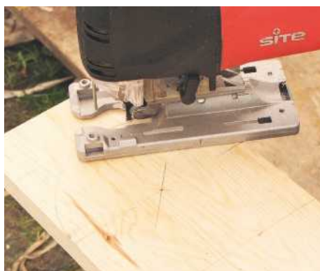
11 Cut around curve with a jigsaw fitted with a narrow blade, keeping to the waste side of the line
