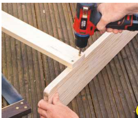
23 Add a stretcher rail across rear uprights for rigidity and strength; fix in place with 5mm screws
